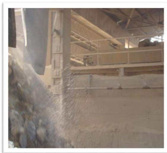
Water spraying System in Crusher Hopper
