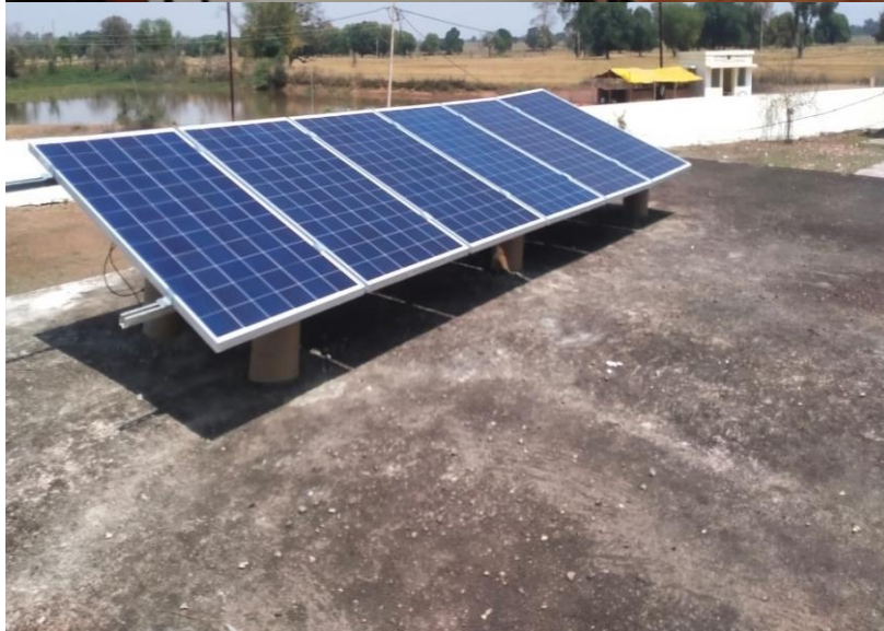
Smart Board with Solar Backup
